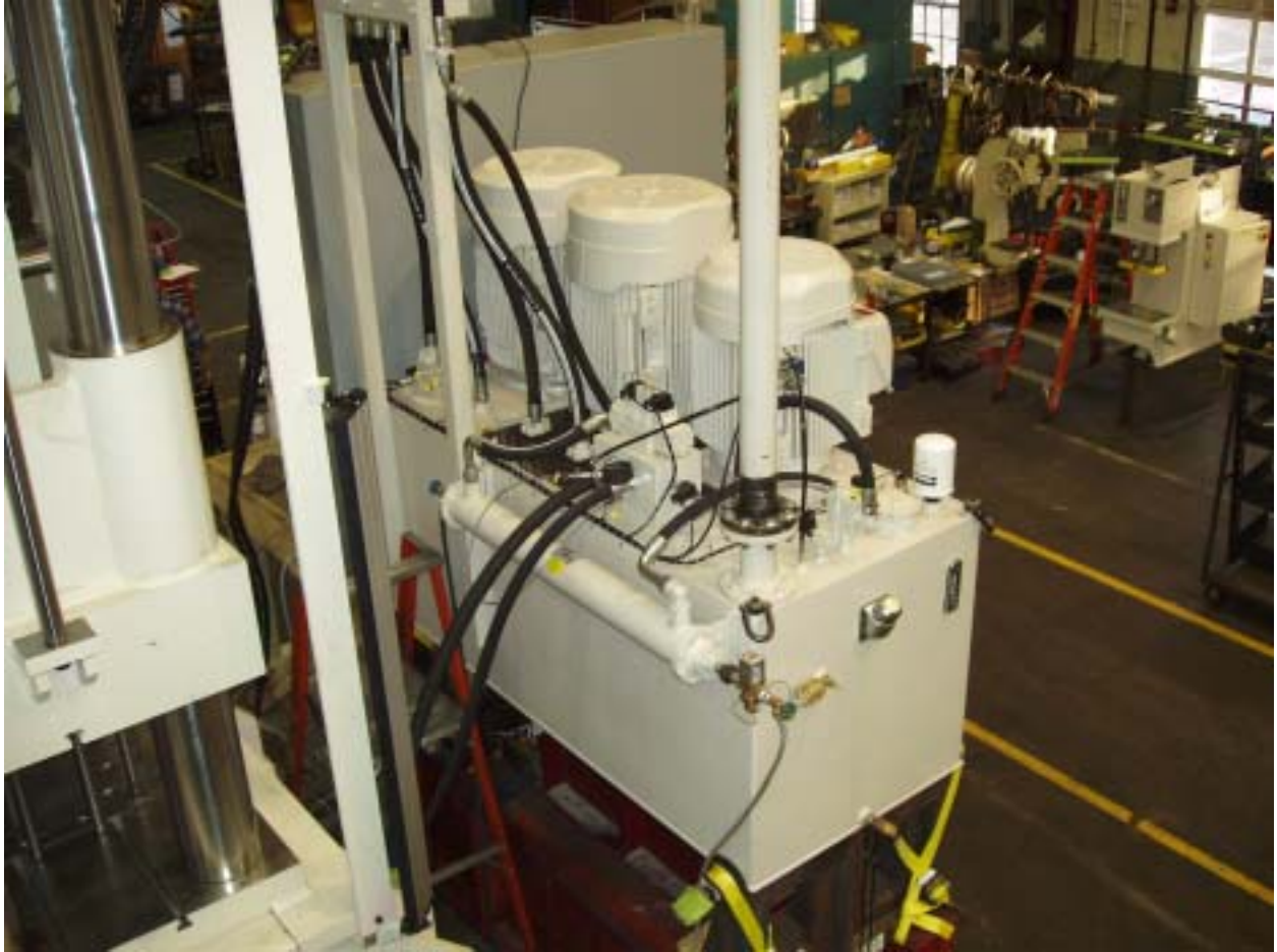
Overhead view of Main Power Unit.
